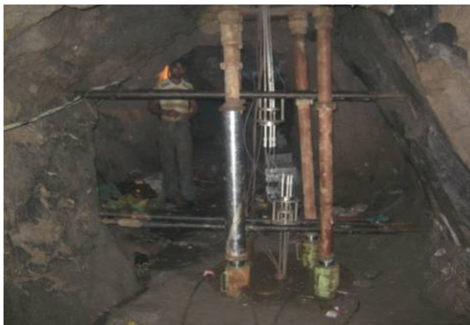
Photograph 2: A Vertical Plate Jacking Test (Vertical Direction) in Progress in Drift at the Project Site
