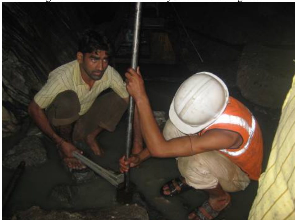
Fig. 7: Rods Being Lowered to Test Depth in Vertical Hole for Hydraulic Fracturing Test
