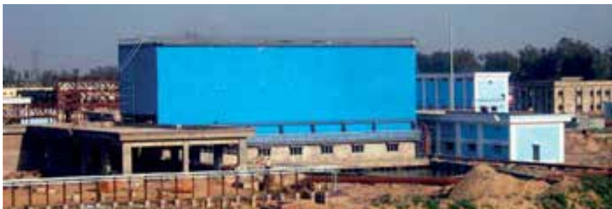
Cooling Water Pump House
