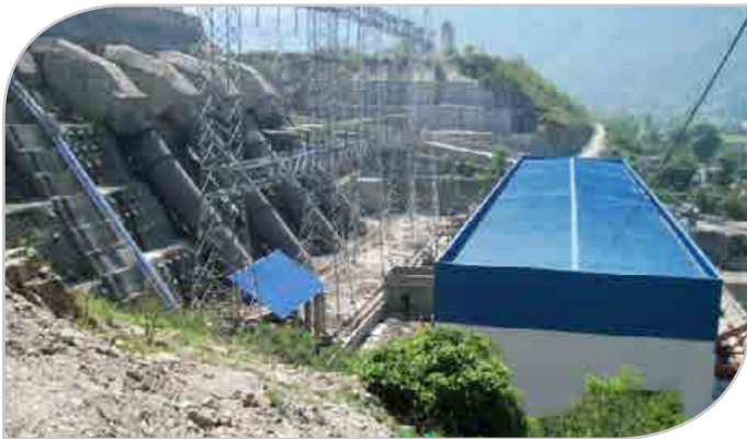
Penstocks of Power House
